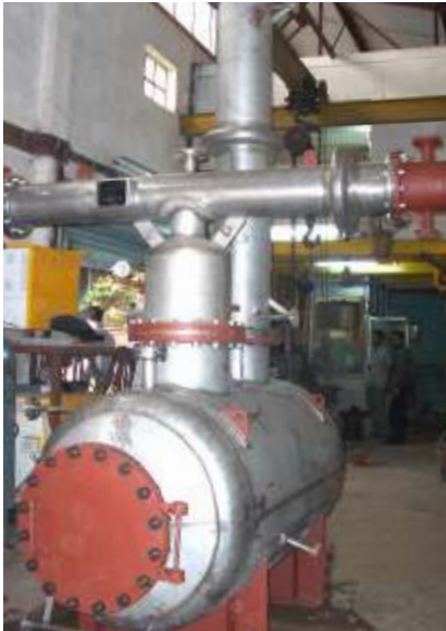
Falling film evaporator & condenser mounted on reboiler Client: Camphor & Allied Products Ltd.
